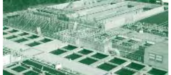
The wash tanks while under construction at the South Parkway Water Treatment Plant.
